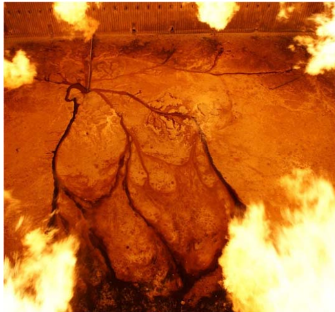
Figure 1. Recovery boiler floor at the end of smelt extraction
